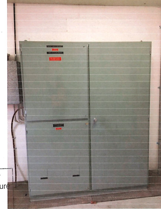
MAIN SWITCH BOARD IN THE SWITCH ROOM
