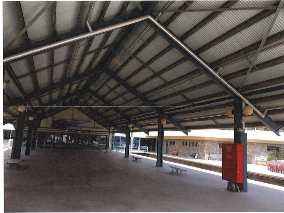
BULLOCKS FLAT TERMINAL PLATFORMS
